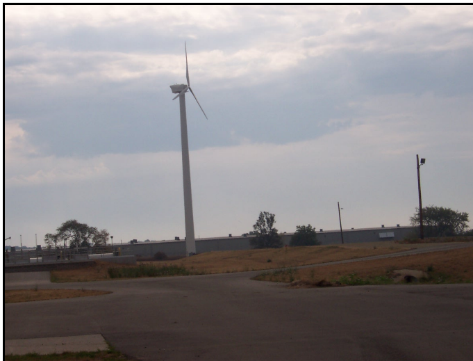
10 KW Wind turbine located at a WWTP Output voltage of 480 volts
